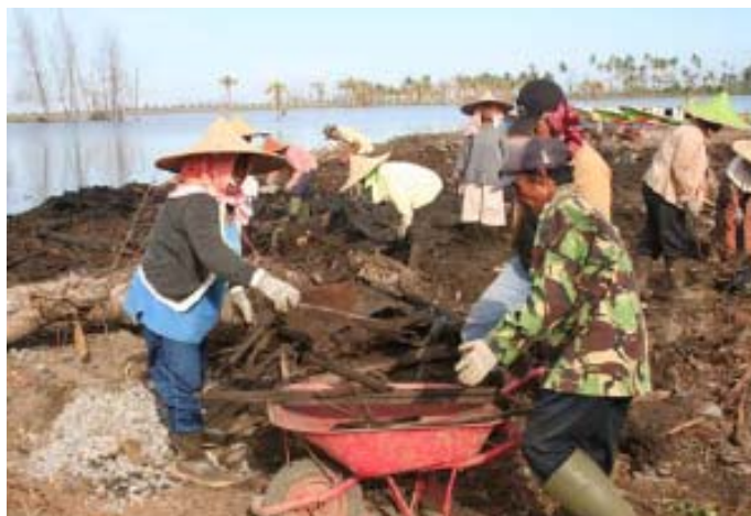
Removal of tsunami waste in Langung temporary dump site in Aceh Barat (Photo: UNDP TRWMP)
